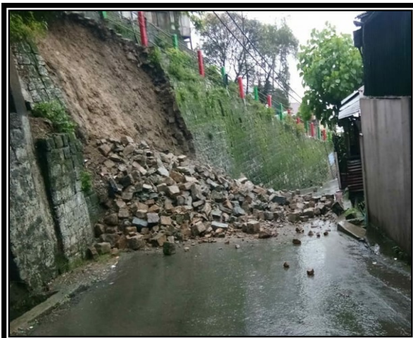
Collapse of retaining wall at Chhinga Veng, Aizawl
