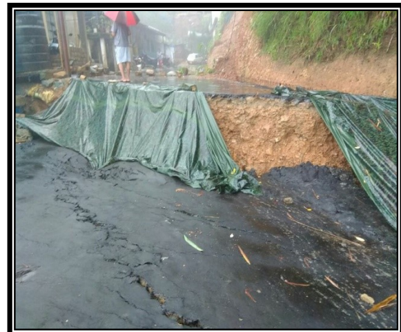
Road damaged at Republic Veng, Aizawl
